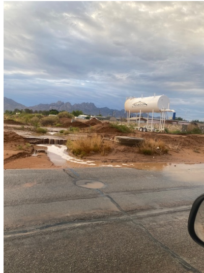
Berm failure on West side of project at Porter Rd. Requires re-establishment and cleaning of fugitive sediment.
